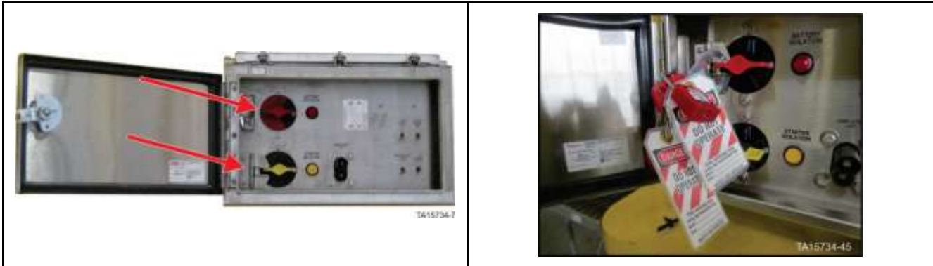
GEN 2 Isolation and Control switches assembly – Battery isolation switch in OFF position with locks in place
