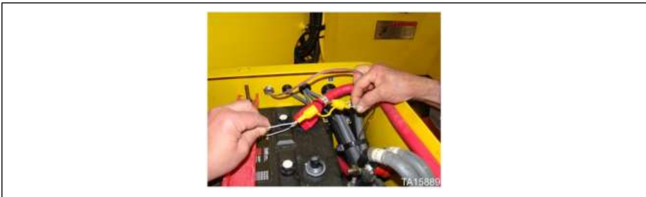
Fire suppression in-line fuse located in loader battery box on some machines
