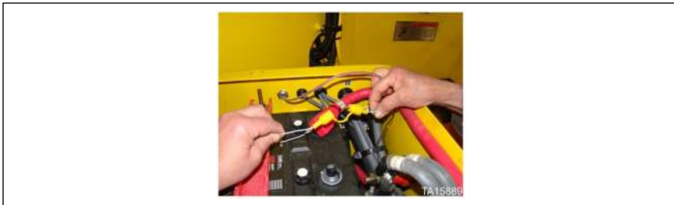
Fire suppression in-line fuse located in loader battery box on some machines
