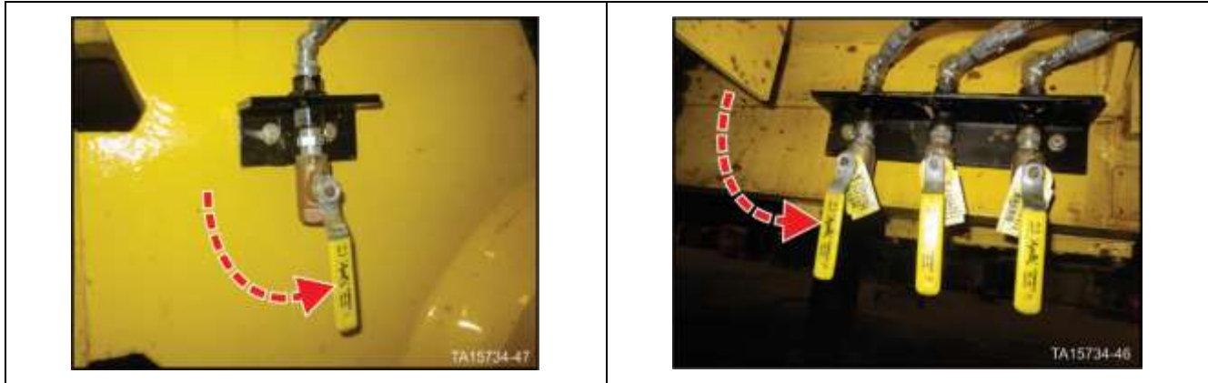
Open air reservoir bleed valves
