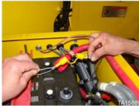
Fire suppression in-line fuse located in loader battery box on some machines
