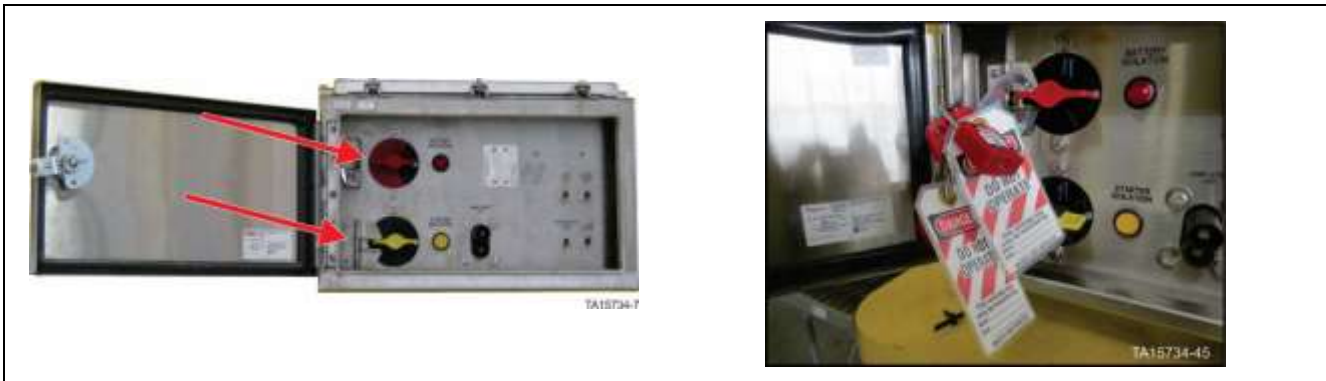
Isolation and Control switches assembly – Battery isolation switch in OFF position with locks in place
