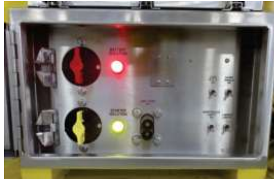
GEN 2 Battery Isolation Box – locks removed – and switches moved to on position
