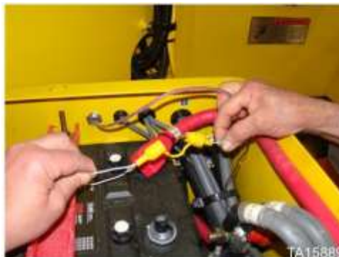
Fire suppression in-line fuse located in loader battery box on some machines
