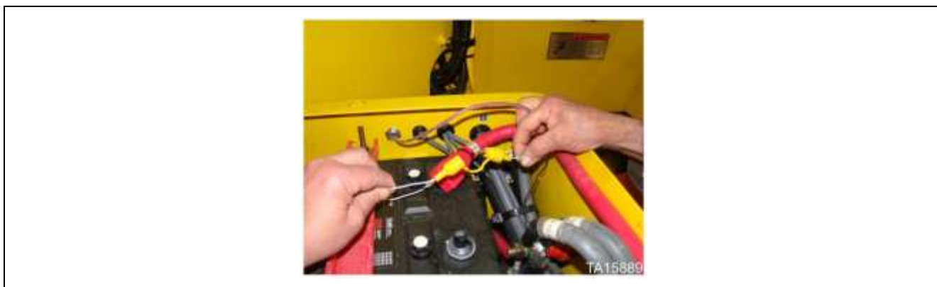
Fire suppression in-line fuse located in loader battery box on some machines
