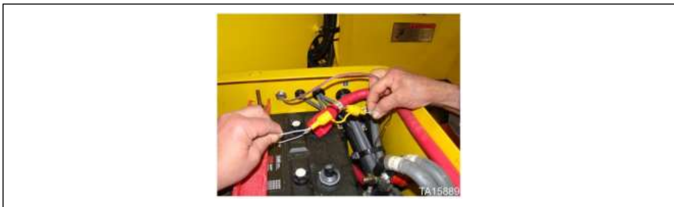
Fire suppression in-line fuse located in loader battery box on some machines
