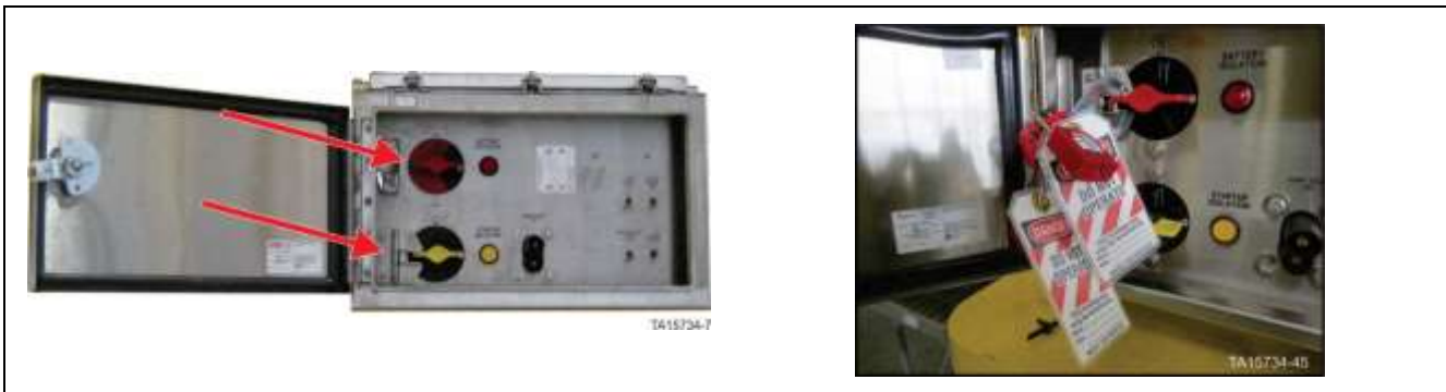
GEN 2 Isolation and Control switches assembly – Battery isolation switch in OFF position with locks in place
