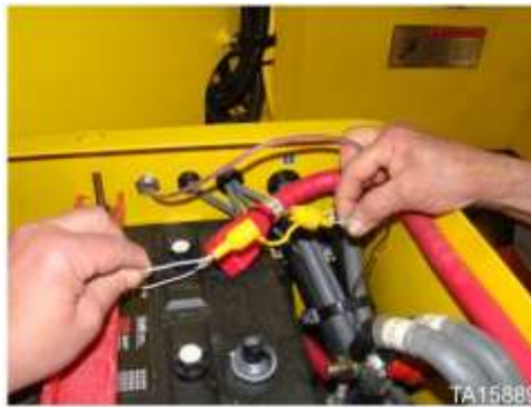
Fire suppression in-line fuse located in loader battery box on some machines
