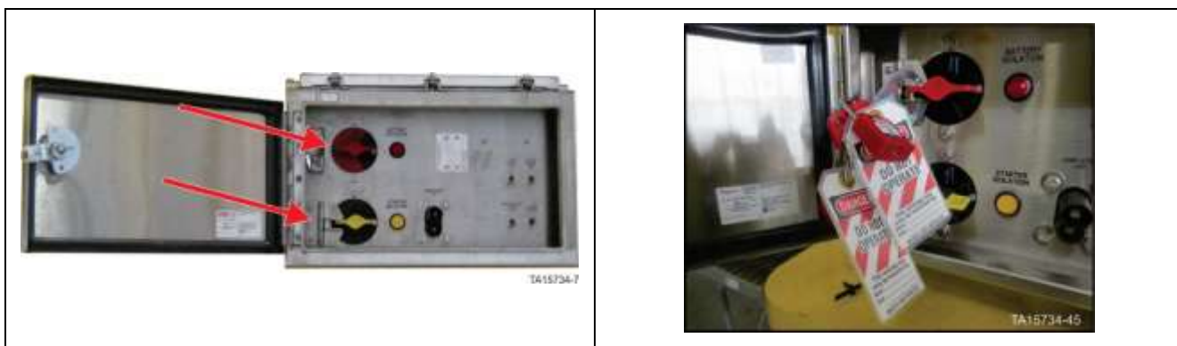
GEN 2 Isolation and Control switches assembly – Battery isolation switch in OFF position with locks in place
