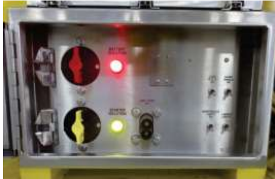
GEN 2 Battery Isolation Box – locks removed – and switches moved to on position
