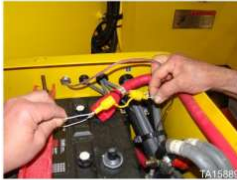
Fire suppression in-line fuse located in loader battery box on some machines
