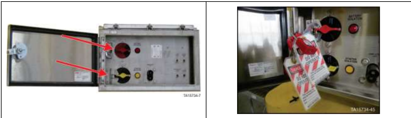
GEN 2 Isolation and Control switches assembly – Battery isolation switch in OFF position with locks in place
