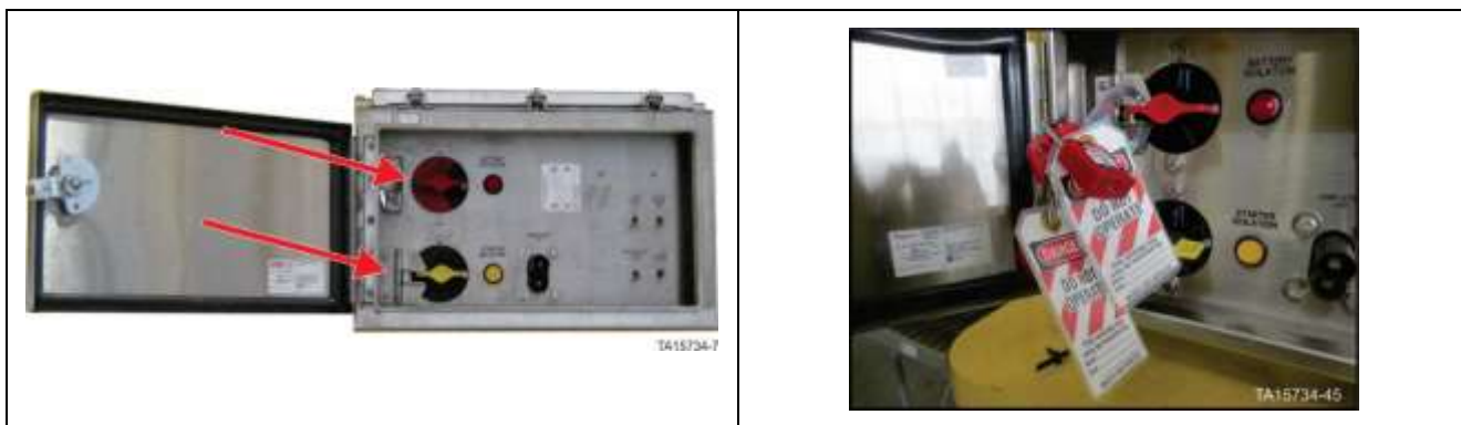
GEN 2 Isolation and Control switches assembly – Battery isolation switch in OFF position with locks in place
