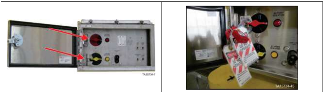
Isolation and Control switches assembly – Battery isolation switch in OFF position with locks in place
