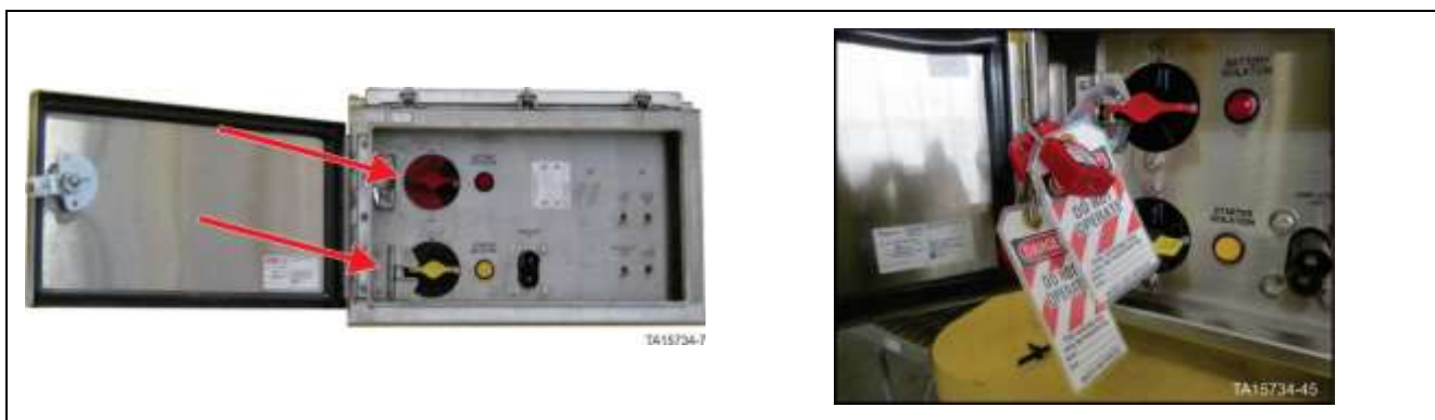
GEN 2 Isolation and Control switches assembly – Battery isolation switch in OFF position with locks in place
