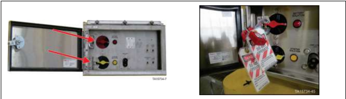
Isolation and Control switches assembly – Battery isolation switch in OFF position with locks in place
