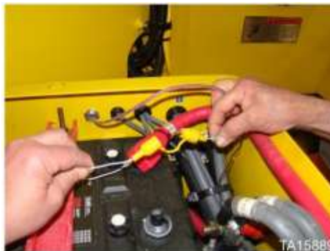
Fire suppression in-line fuse located in loader battery box on some machines
