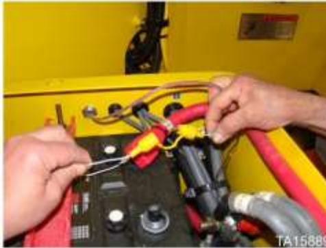
Fire suppression in-line fuse located in loader battery box on some machines
