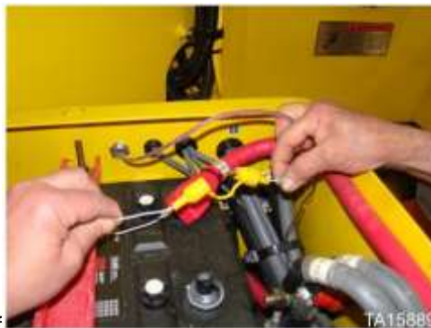
Fire suppression in-line fuse located in loader battery box on some machines
