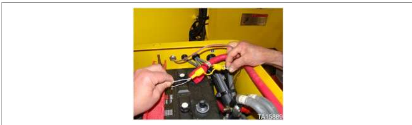
Fire suppression in-line fuse located in loader battery box on some machines
