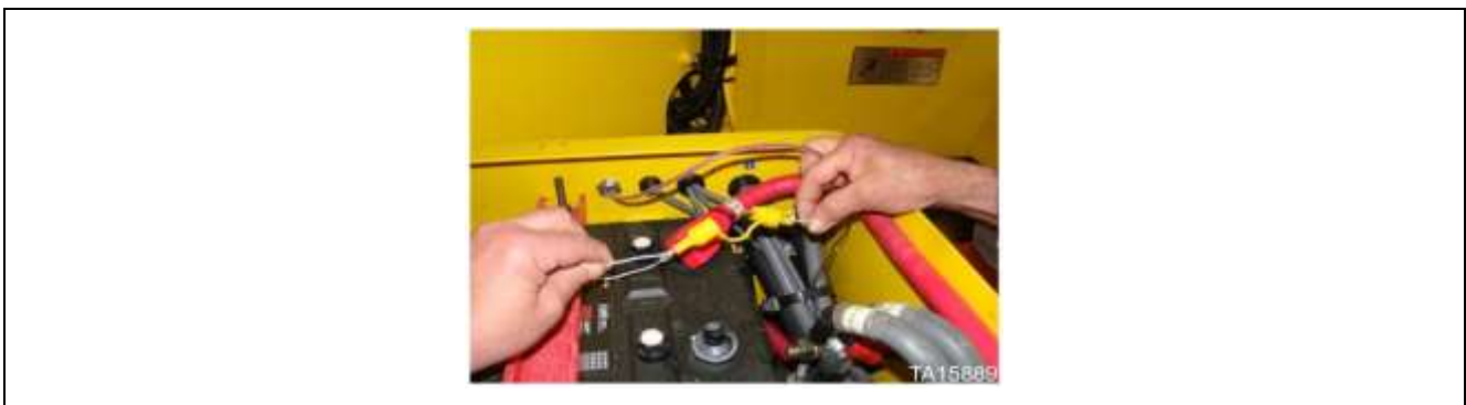
Fire suppression in-line fuse located in loader battery box on some machines
