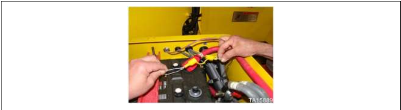
Fire suppression in-line fuse located in loader battery box on some machines
