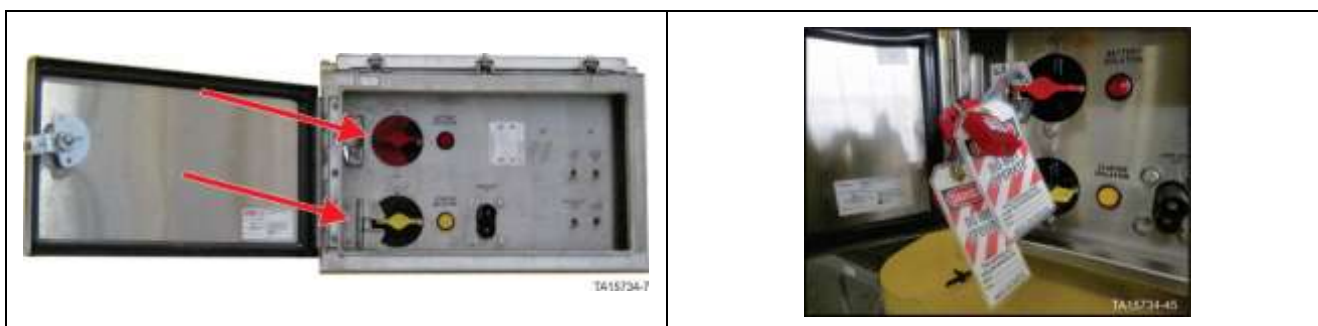
GEN 2 Isolation and Control switches assembly – Battery isolation switch in OFF position with locks in place
