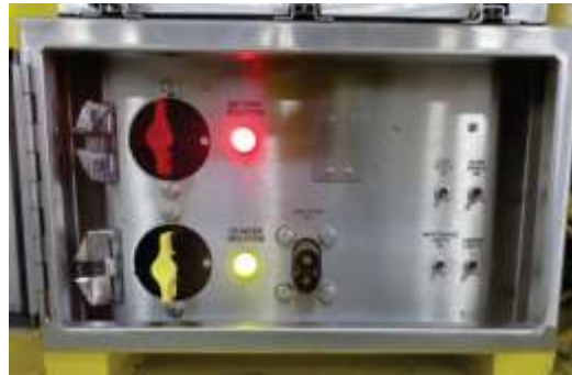
GEN 2 Battery Isolation Box – locks removed – and switches moved to on position
