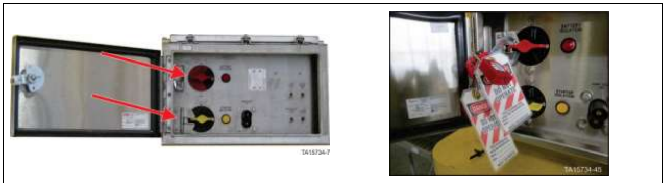
Isolation and Control switches assembly – Battery isolation switch in OFF position with locks in place
