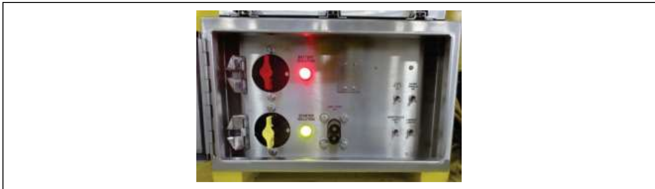
GEN 2 Battery Isolation Box – locks removed – and switches moved to on position
