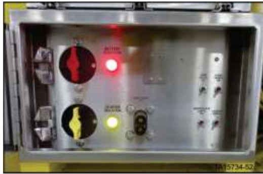
GEN 2 Battery Isolation Box – locks removed – and switches moved to on position
